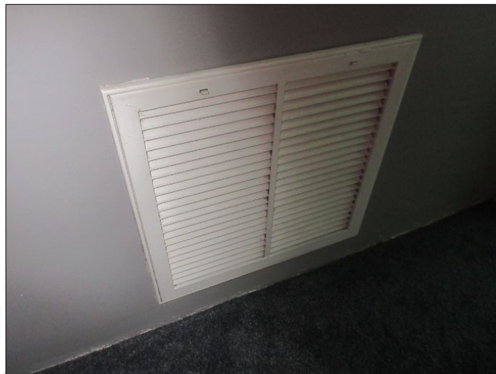
HVAC Return 2nd fl
