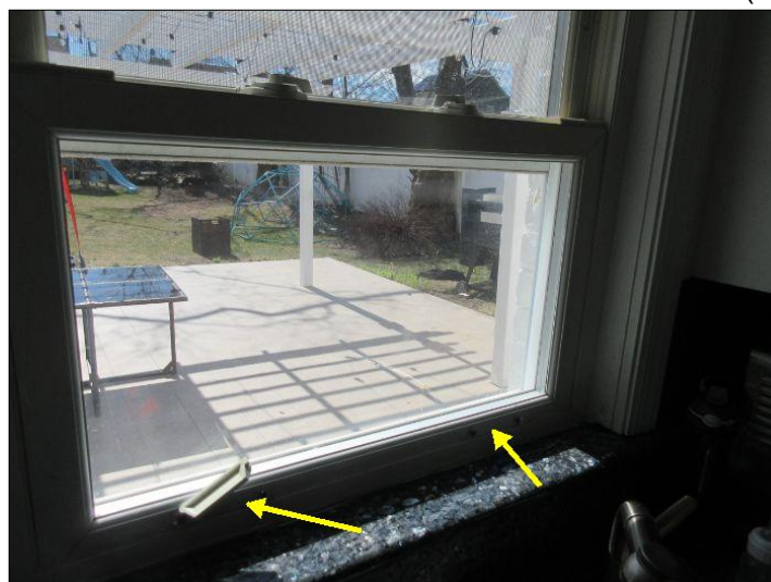
Damaged hardware noted (Kitchen)
