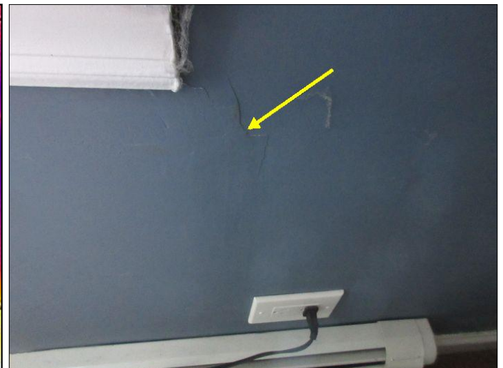
Wall repair noted - Damage from shifting foundation. Coincides w/ cracks at front brick veneer (Bedroom #5)
