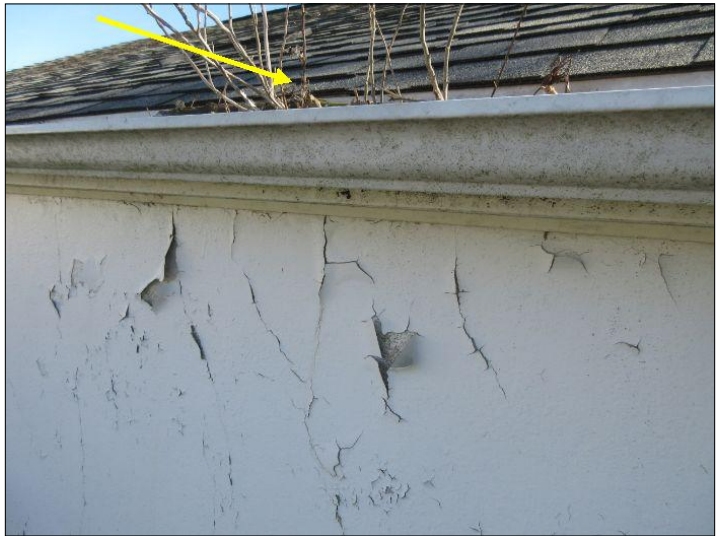
Areas of gutters clogged
