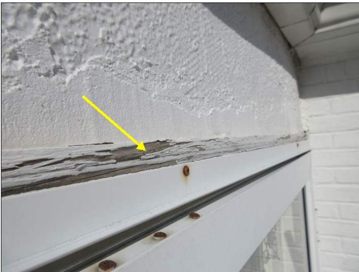
Deteriorated materials noted (Rear door)
