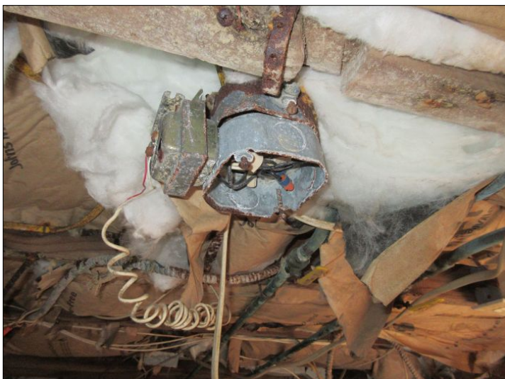
Missing junction box cover. Repair as needed. (Crawlspace)
