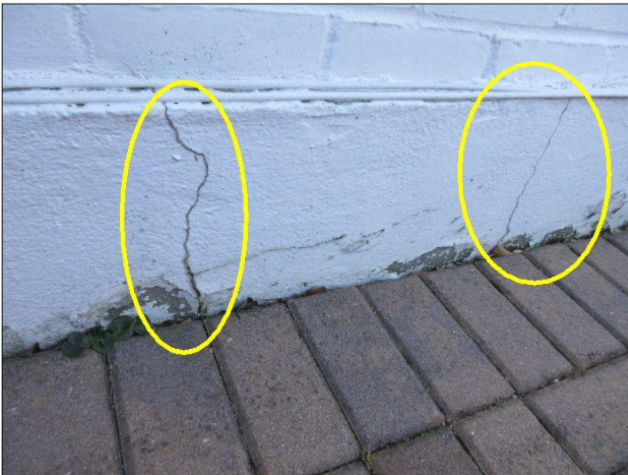
Minor cracking noted (Right side)
