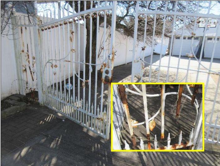
Driveway gate showing signs of deterioration. Recommend budgeting for replacement.
