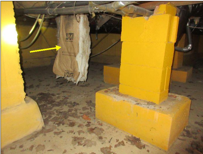
Insulation loose in area(s)
