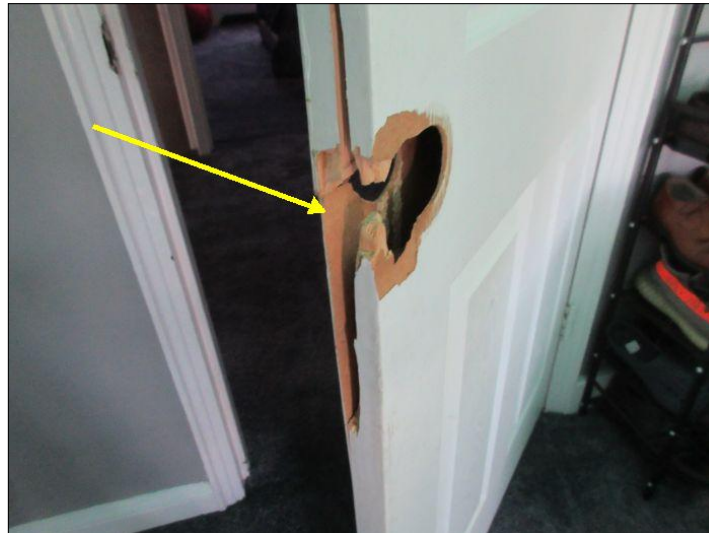
Damaged door, replacement required (Bedroom #3)
