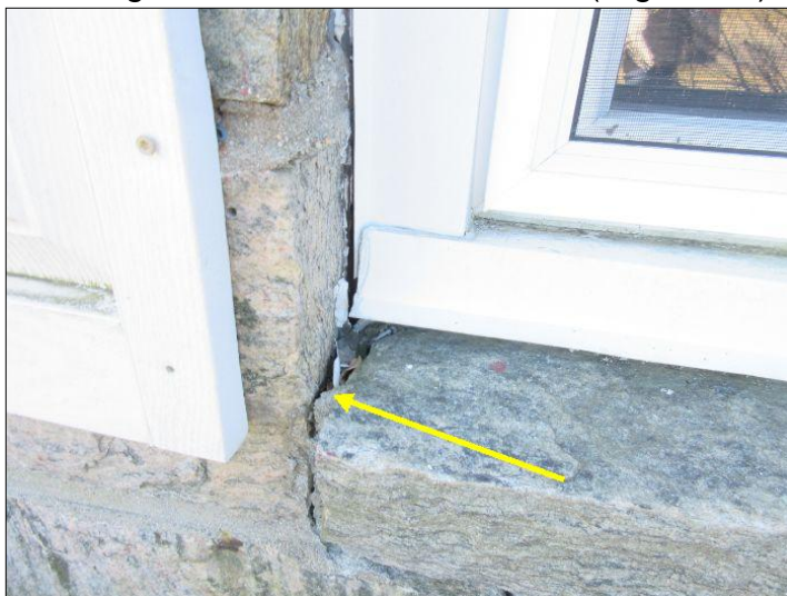
Structural crack noted at front of home. Result from undermining of foundation.
