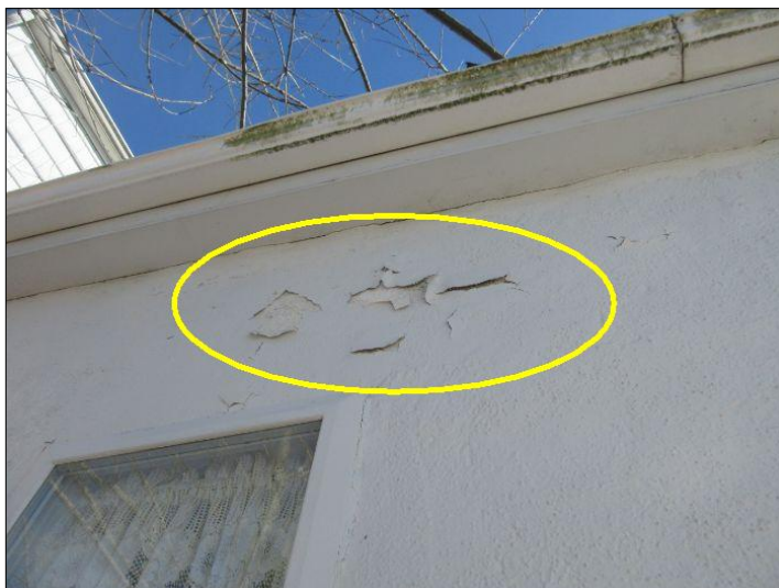
Flaking noted. Refinish as needed (Right side)
