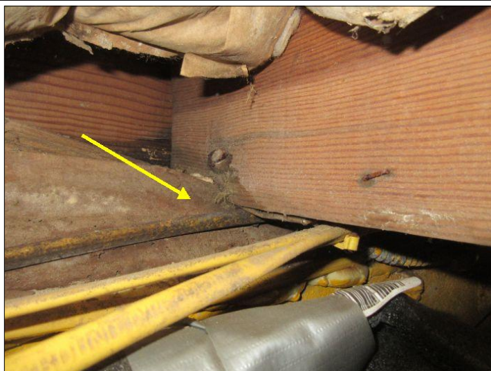
Damaged sill plate
