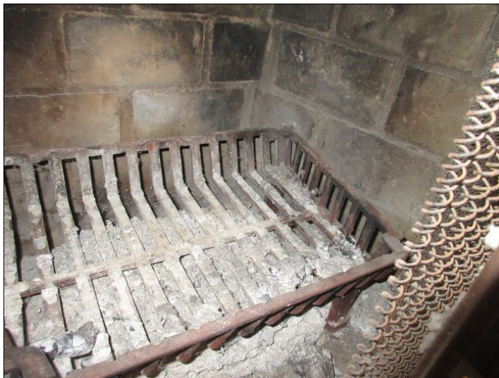
Recommend cleaning (Master Bedroom)
