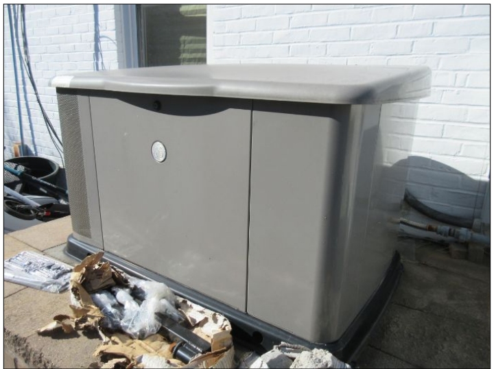
Backup generator - Locked, unable to test
