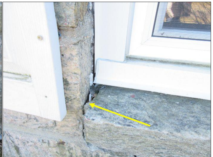
Structural crack noted at front of home. Result from undermining of foundation.
