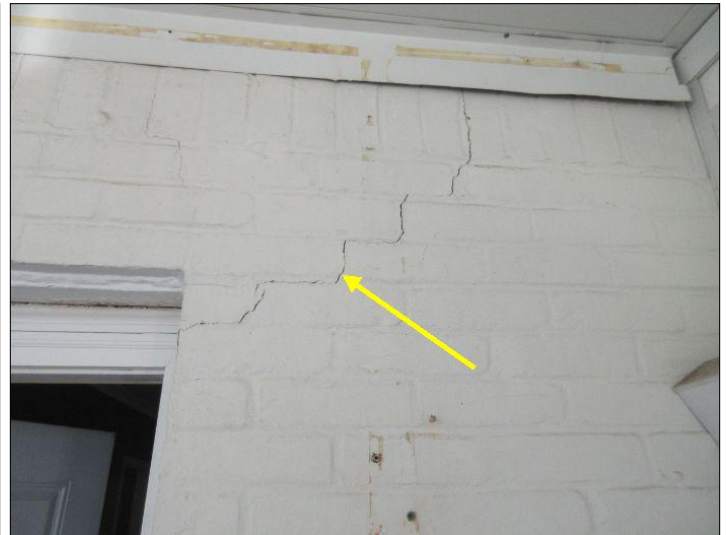
Step cracking noted - Related to damaged sill plate (Rear)
