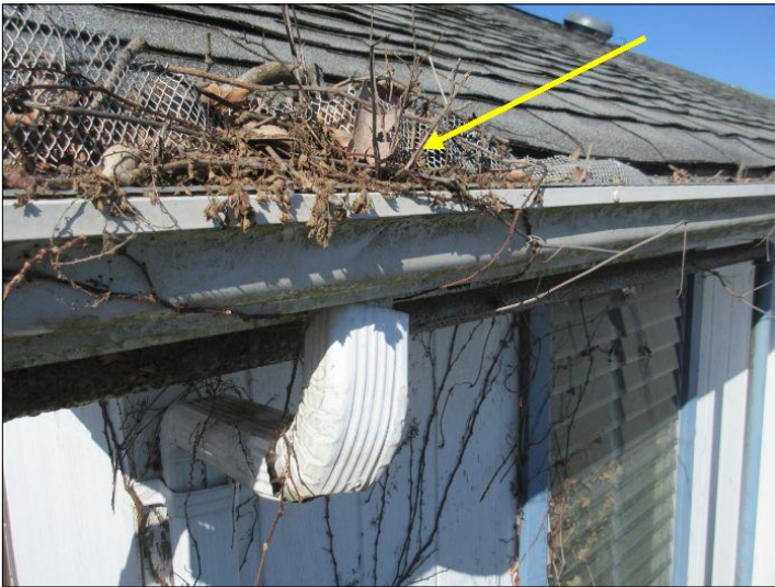
Areas of gutters clogged
