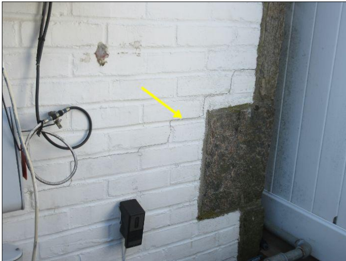
Additional cracks coinciding w/ undermined foundation
