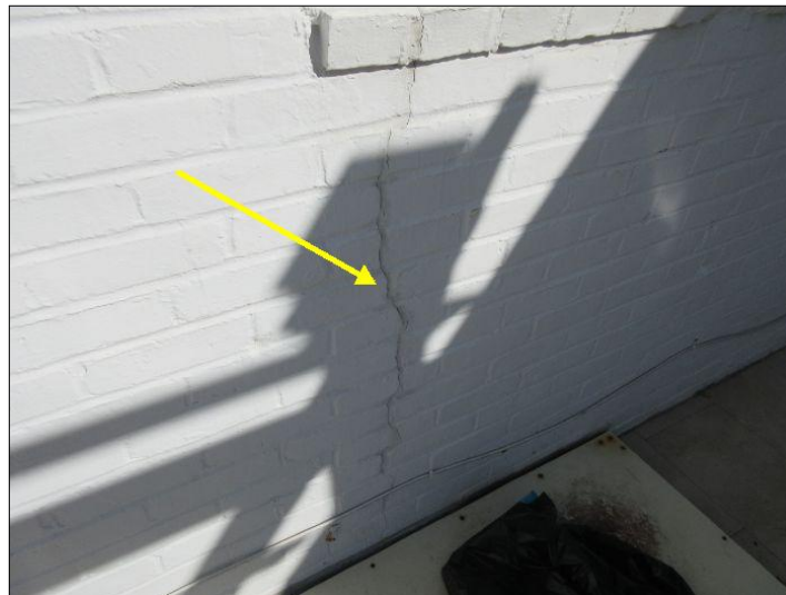
Cracking noted - Likey caused by deteriorated sill plates at rear of home
