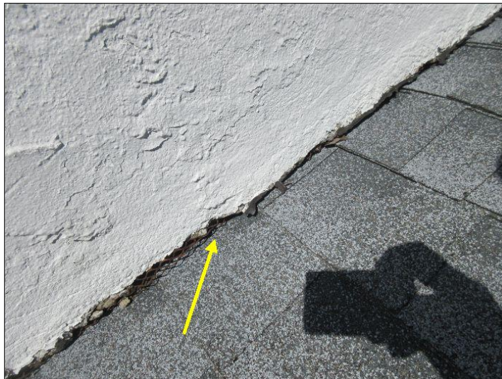
Recommend installing of step flashing to prevent water penetration
