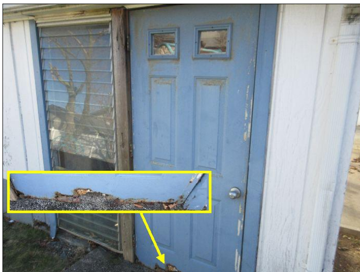
Side door deteriorated - Requires replacement
