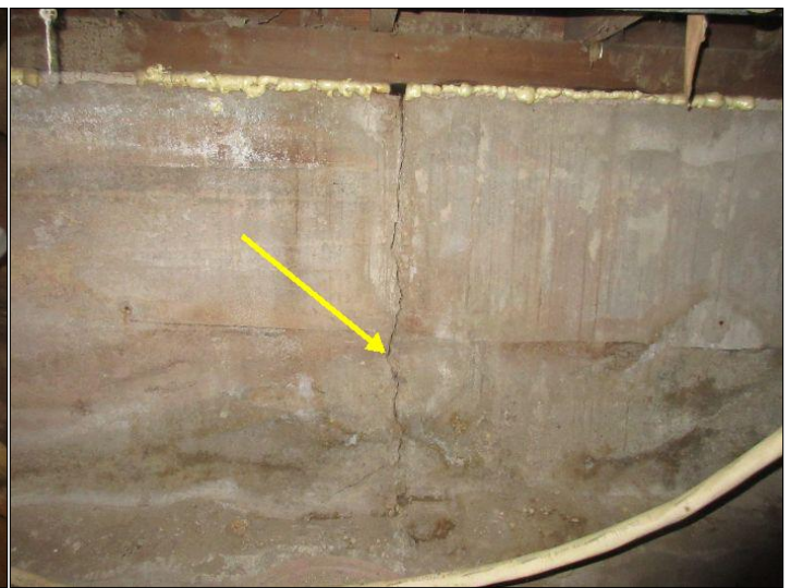
Crack at front wall extends to base of foundation
