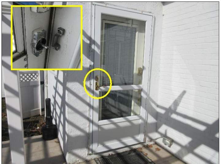
Missing hardware noted
