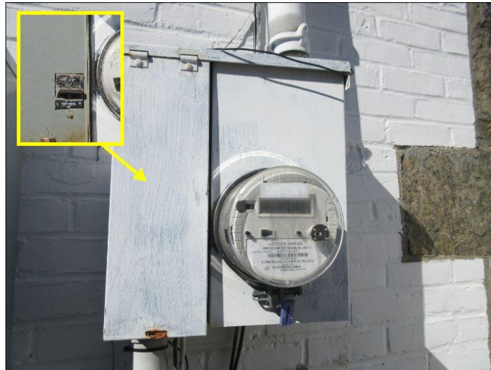
Main service disconnect
