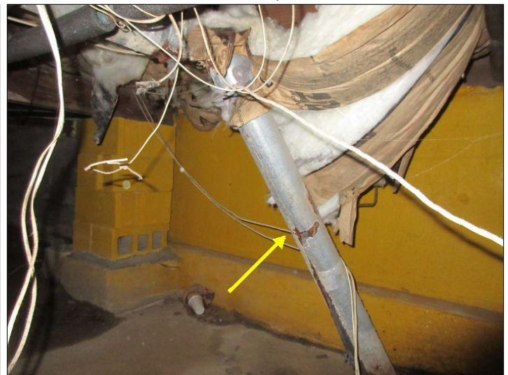
Dryer vent has failed and collapsed
