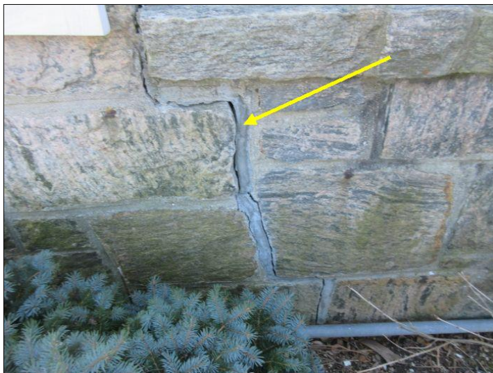
Structural crack noted at front of home. Result from undermining of foundation.
