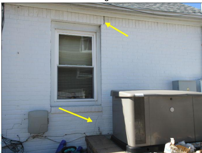
Additional cracks coinciding w/ undermined foundation
