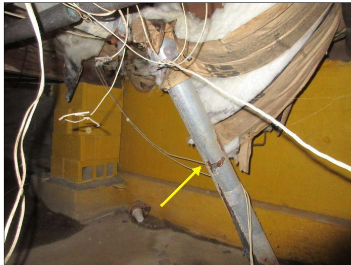
Dryer vent has failed and collapsed
