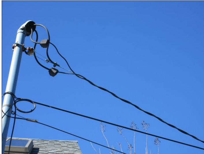
Electrical service mast
