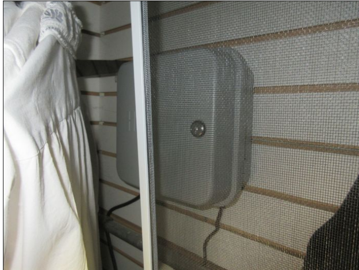
Sprinkler system timer (Utility Room)
