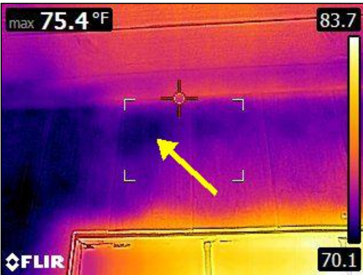
Indications of water penetration in cedar closet (Thermal View)
