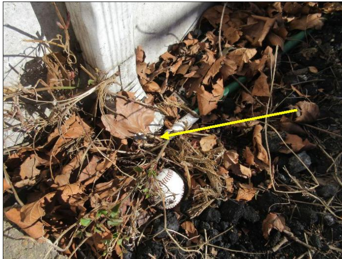
Discharge blocked. Clear as needed (Rear)
