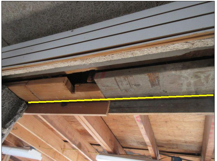
Structural - Missing header noted at opening in rear of garage
