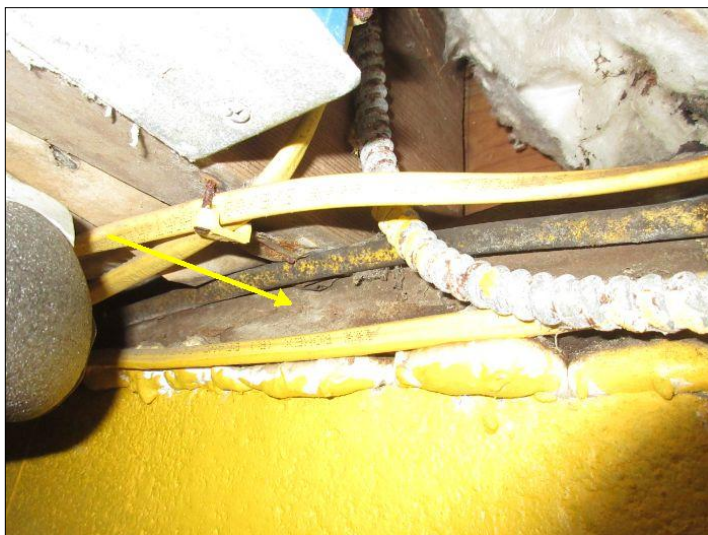
Damaged sill plate
