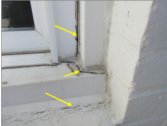
Gaps noted at rear window trim - Additional results from rear sill plate deterioration
