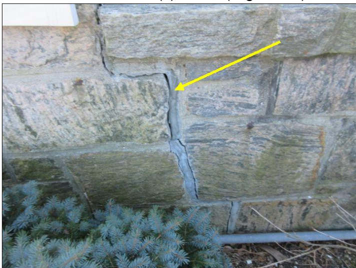
Structural crack noted at front of home. Result from undermining of foundation.
