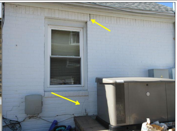
Additional cracks coinciding w/ undermined foundation
