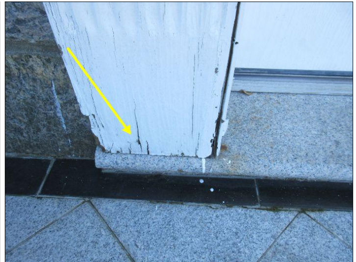
Deteriorated materials noted (Front door)
