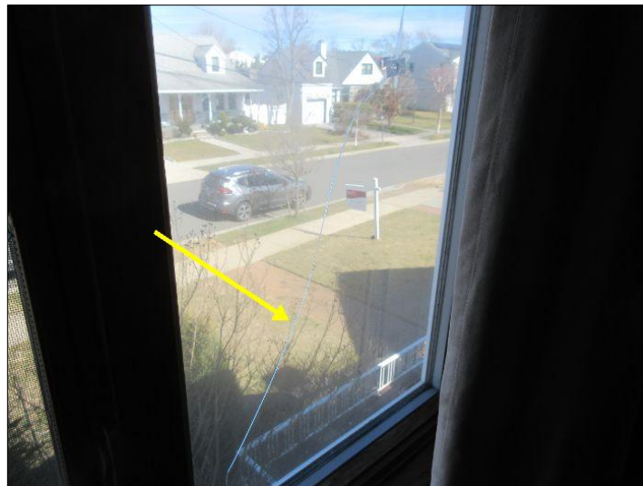
Broken glass (Master Bedroom)
