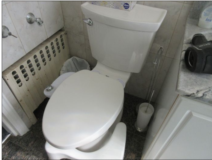
Operated when tested. No deficiencies noted.
