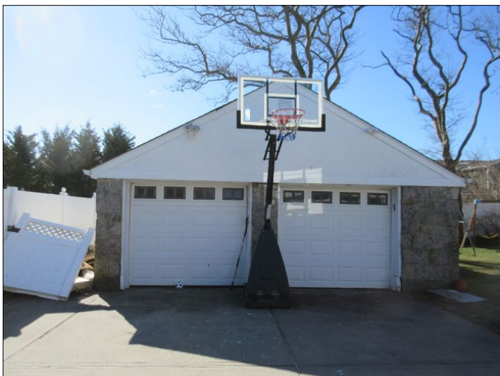
Not tested due to stored items behind doors
