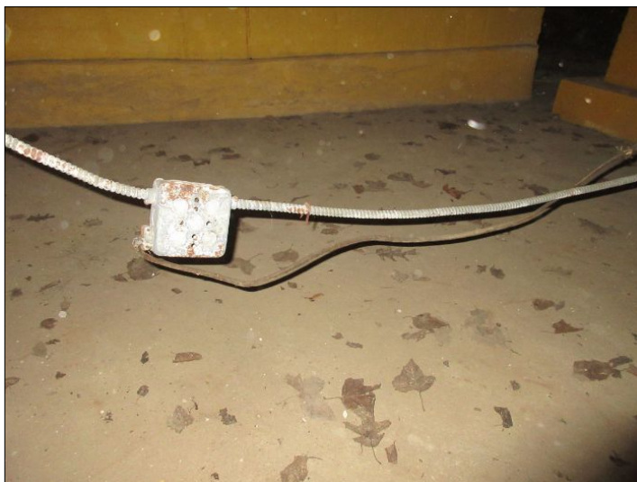
Recommend securing wires as needed (Crawlspace)
