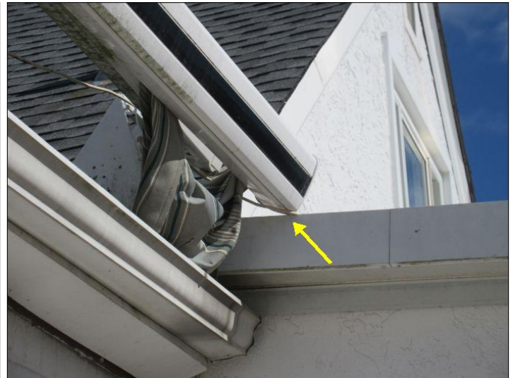
Rear awning rubs against roof. Does not operate correctly.
