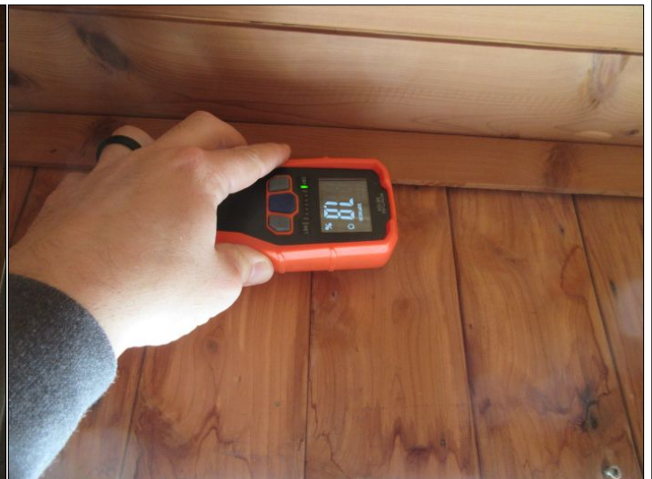
Higher moisture content verified w/ moisture meter
