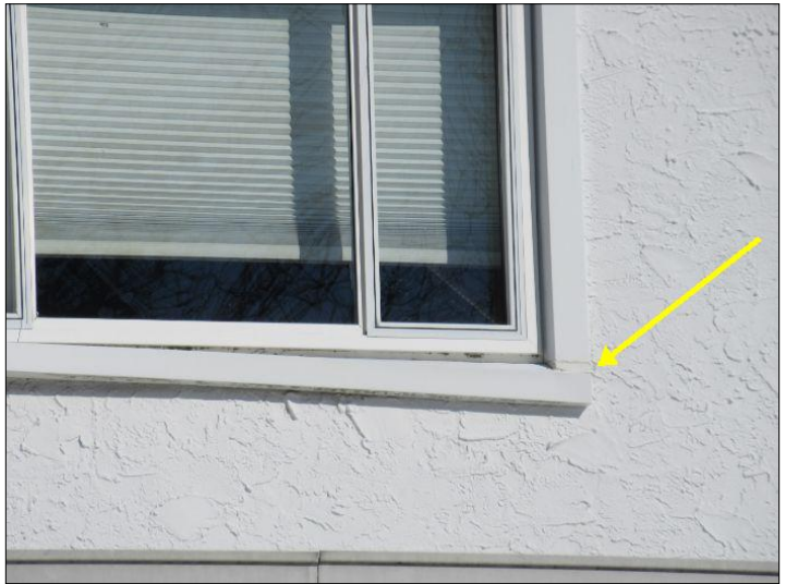
Loose / Sagging trim noted (2nd floor rear)
