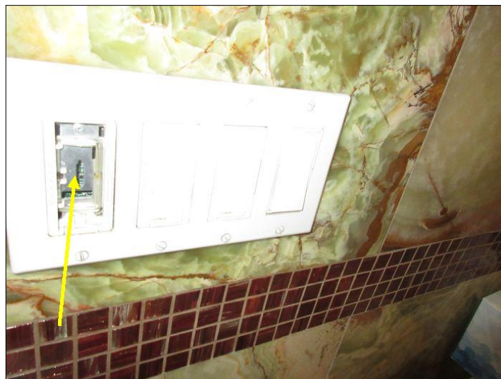
Damaged switch noted. Replace as needed (Bathroom #1)
