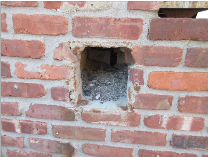
Cleanout cover missing (Right side)
