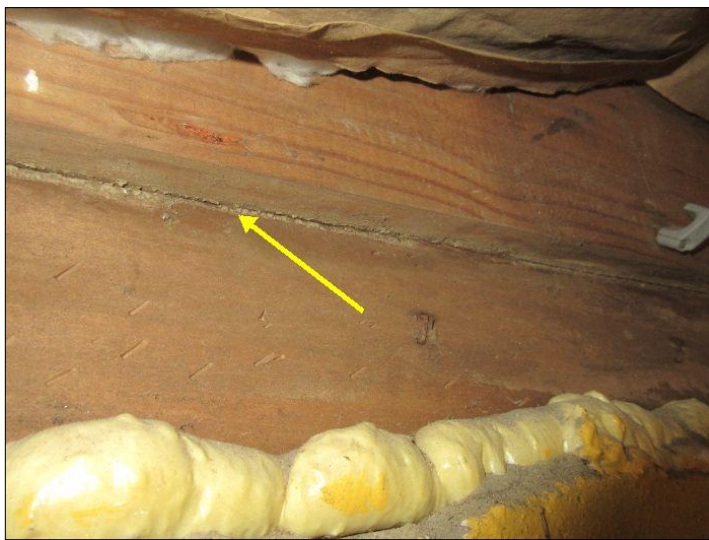
WDO evidence noted at sill plates
