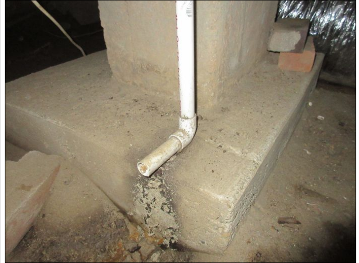
1st floor - Condensation drips into dirt floor in crawlspace, creating a more humid environment. Recommend installation of condensation pump to direct water out of home.
