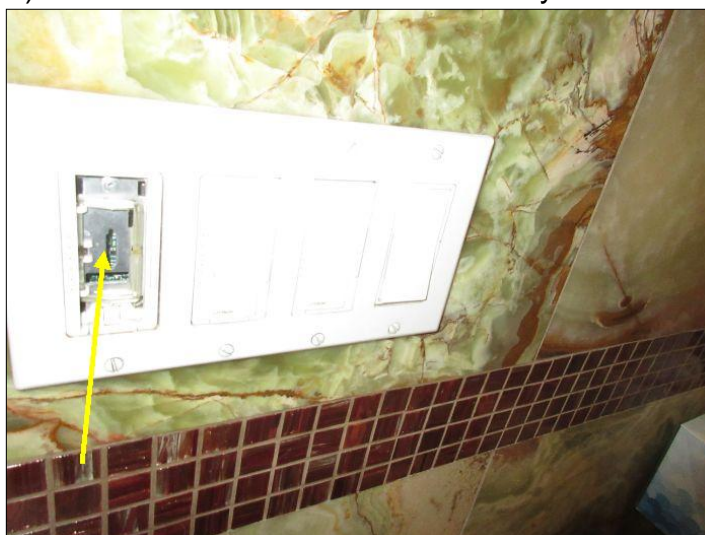
Damaged switch noted. Replace as needed (Bathroom #1)
