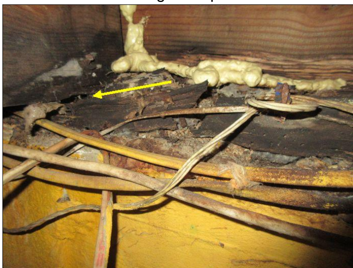
Damaged sill plate
