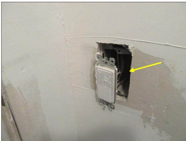
Loose switch noted, recommend correction as needed by licensed electrician (2nd fl closet)
