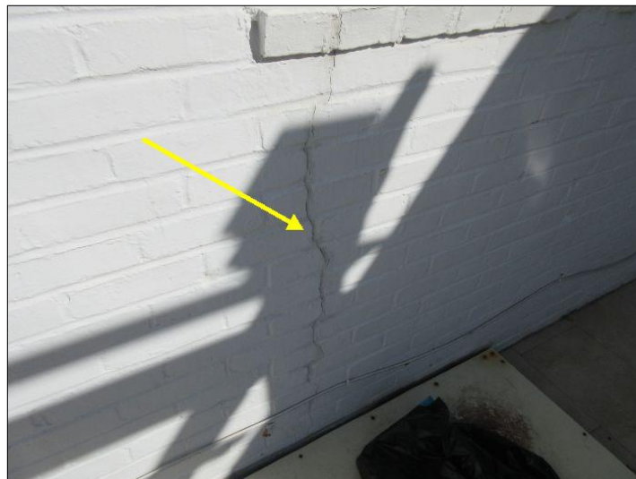
Cracking noted - Likey caused by deteriorated sill plates at rear of home
