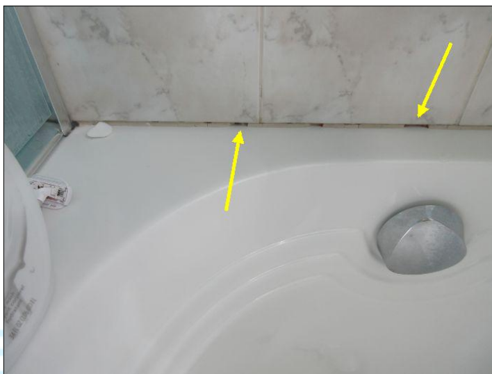
Some grout repair needed
