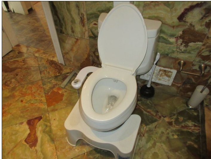
Operated when tested. No deficiencies noted.
