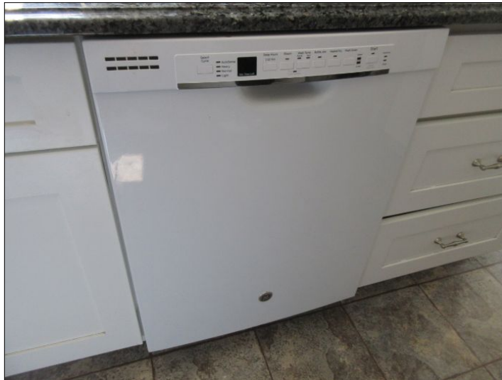
Not Inspected - Personal items in machine.
