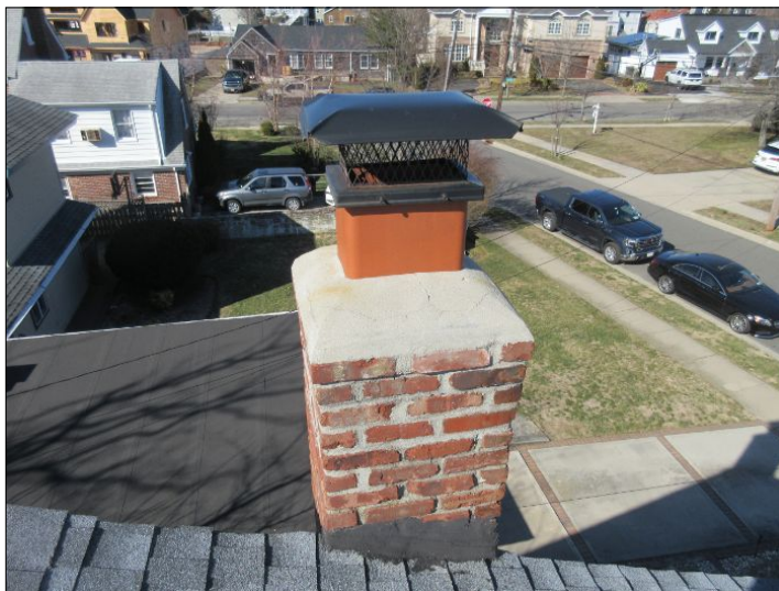
Appeared functional at time of inspection (Bedroom Fireplace)
