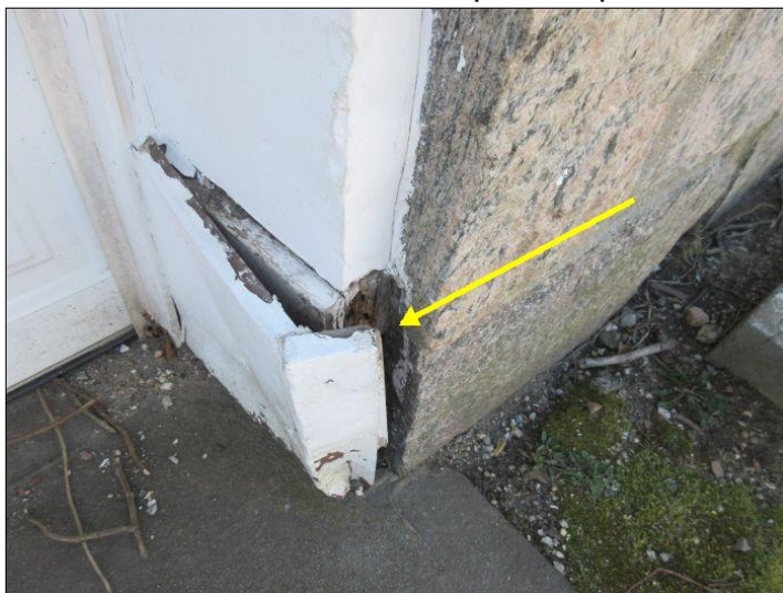
Deteriorated trim noted
