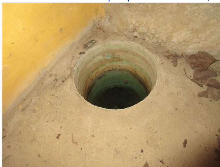
Catch basin noted. Recommend installation of pump to remove water, as needed.
