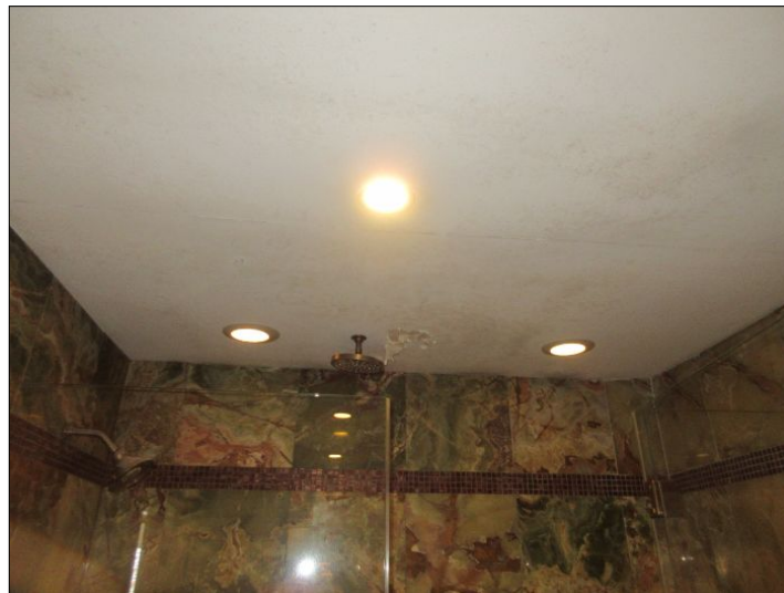
Mold like bio growth stains observed. Professional testing and evaluation is advised. Repair as needed.
