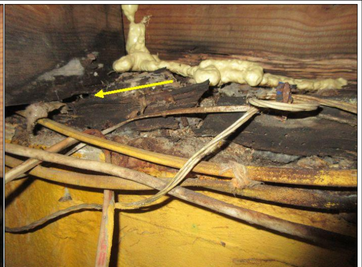
Damaged sill plate
