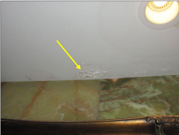
Evidence of active leak noted, likely from missing step flashing (Bathroom #1)
