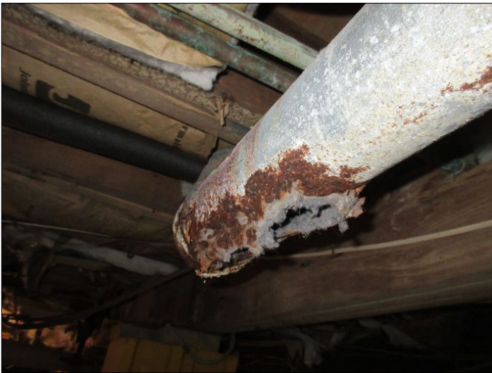
The dryer vent duct has failed and the dryer exhaust vents into the crawlspace
