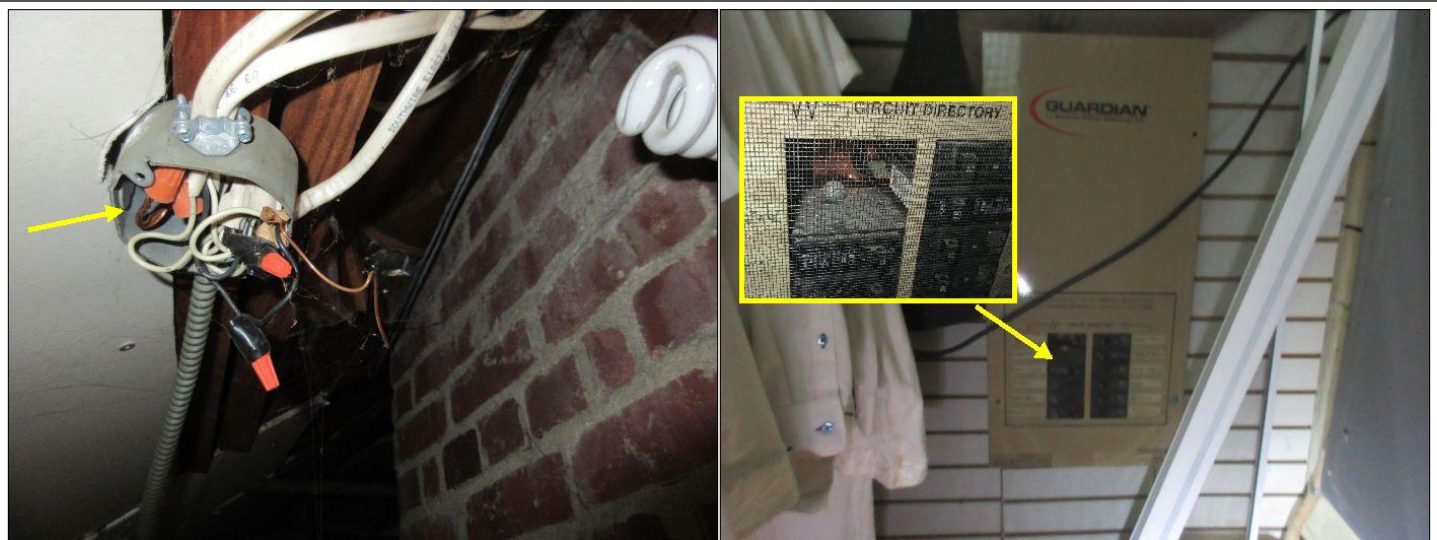
Missing junction box cover (2nd fl hallway closet) Backup Generator Circuit Box - Open knockouts noted, secure as needed
