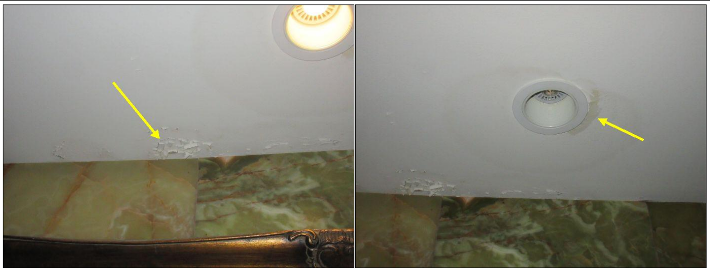
Evidence of active leak noted, likely from missing step flashing (Bathroom #1)
