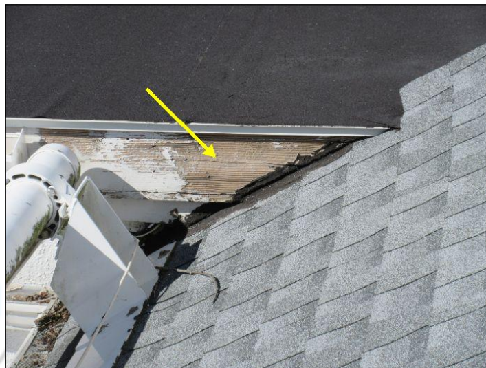
Weathered wood noted. Recommend correction as needed (Rear)
