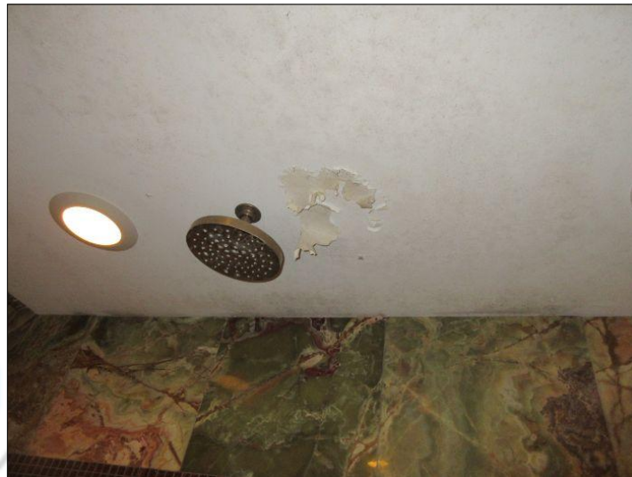
Mold-like bio growth observed. Professional testing & evaluation advised (Bathroom #1)
