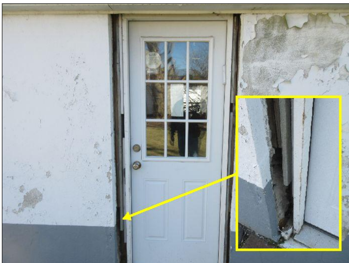
Exterior trim missing
