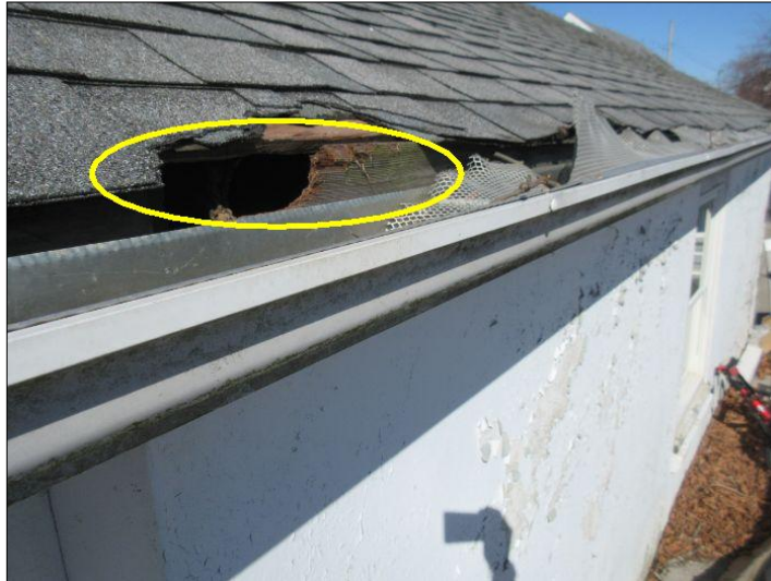
Damaged area(s) noted - Likely area of pest entrance
