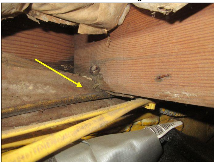
Damaged sill plate
