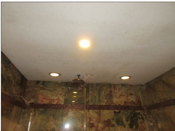
Mold like bio growth stains observed. Professional testing and evaluation is advised. Repair as needed.
