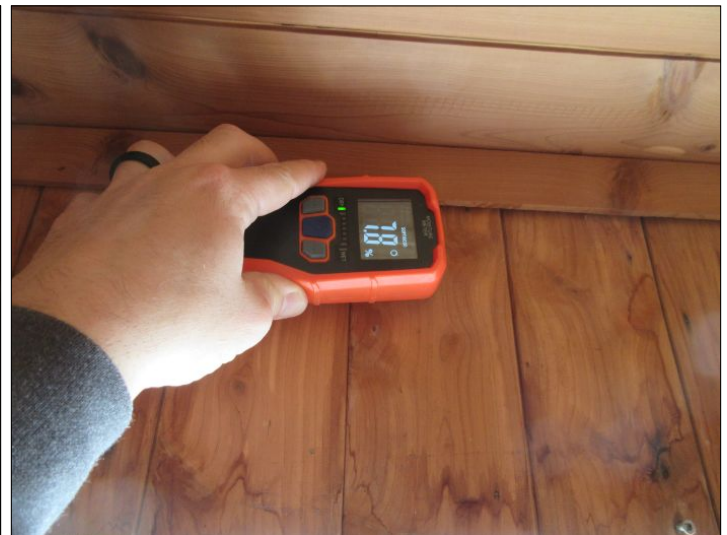
Higher moisture content verified w/ moisture meter
