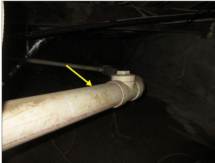
Recommend additional supports as needed
