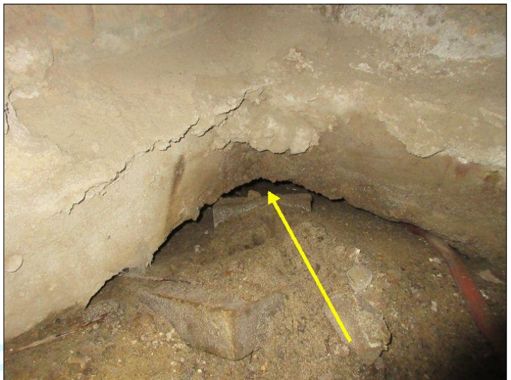
Undermining noted at front left corner of the home's foundation wall.
