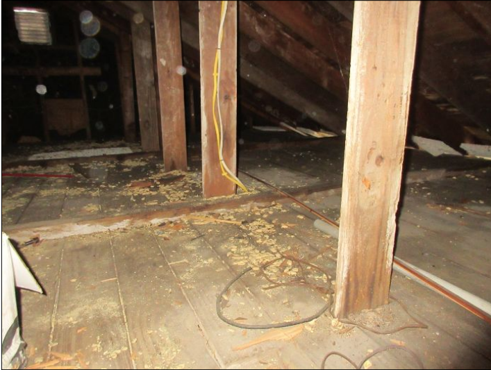
Front area - Viewed from access hole. Visible areas appeared satisfactory. Evidence of previous pest intrusion. Recommend garage is sealed to prevent further pest intrusion.
