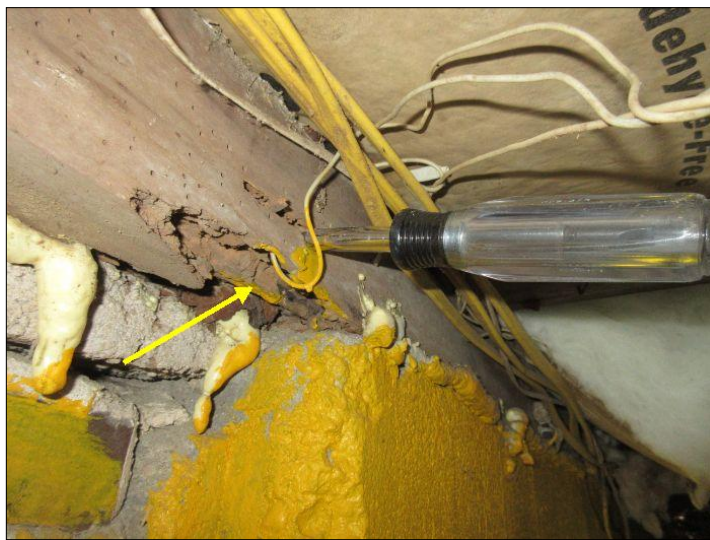
WDO damaged sill plate (Rear wall)
