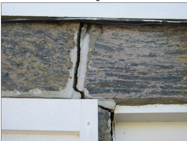
Structural crack noted at front of home. Result from undermining of foundation.
