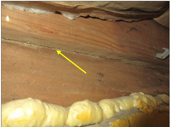
WDO evidence noted at sill plates
