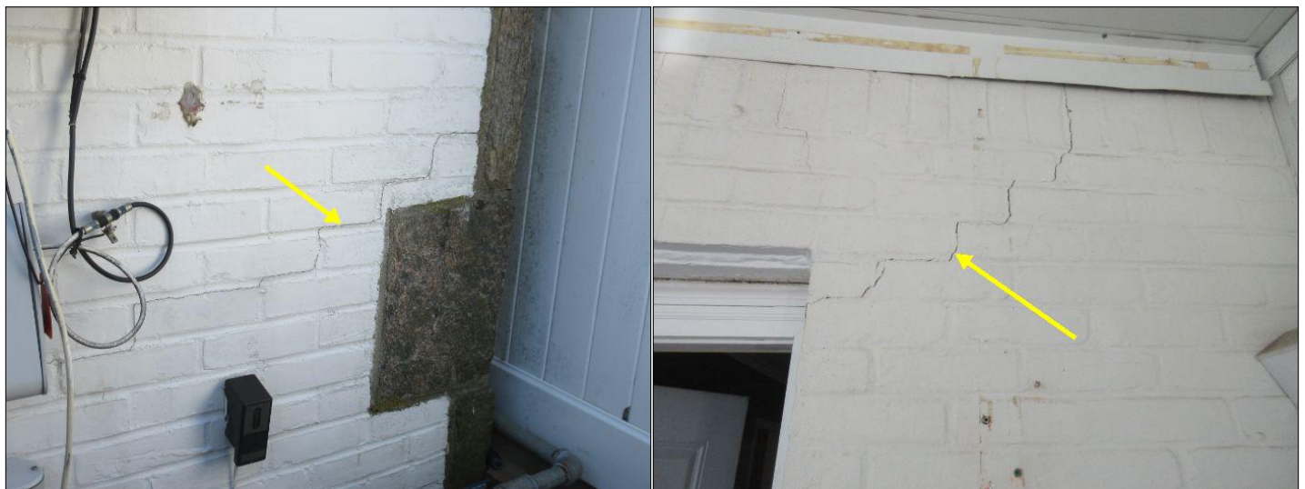
Additional cracks coinciding w/ undermined foundation
