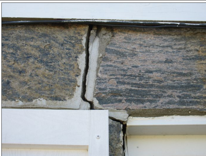
Structural crack noted at front of home. Result from undermining of foundation.
