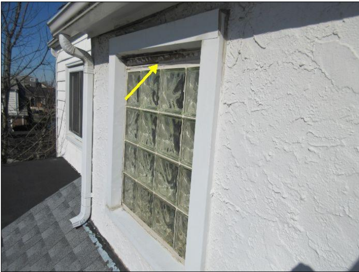
Exposed wood surfaces observed. Recommend enclosing as needed.
