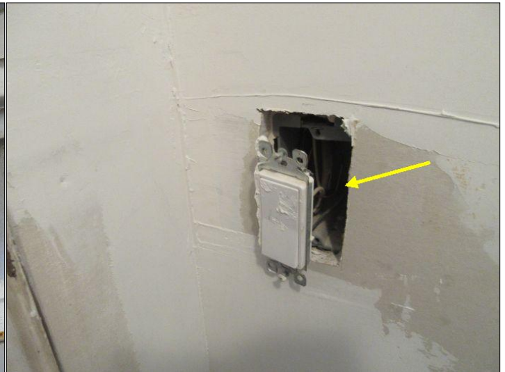
Loose switch noted, recommend correction as needed by licensed electrician (2nd fl closet)
