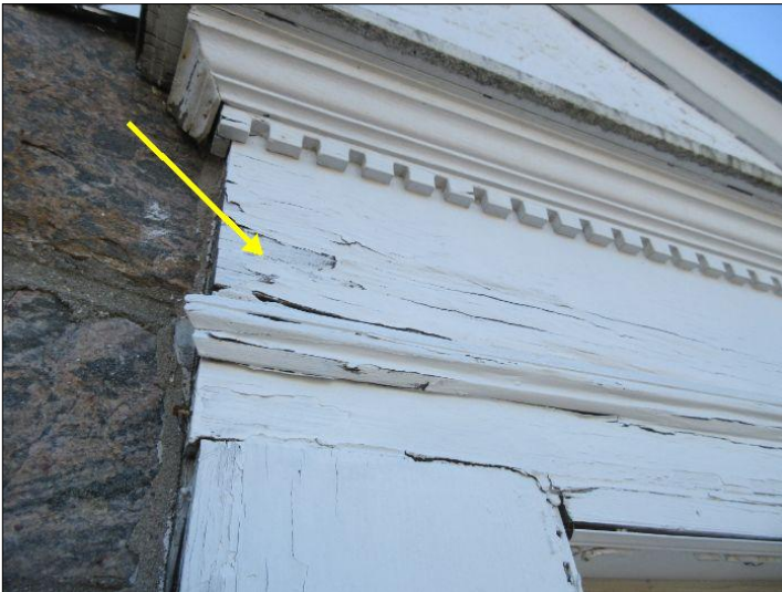
Deteriorated materials noted (Front door)
