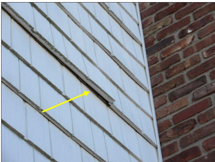
Loose material(s) noted (Right side)
