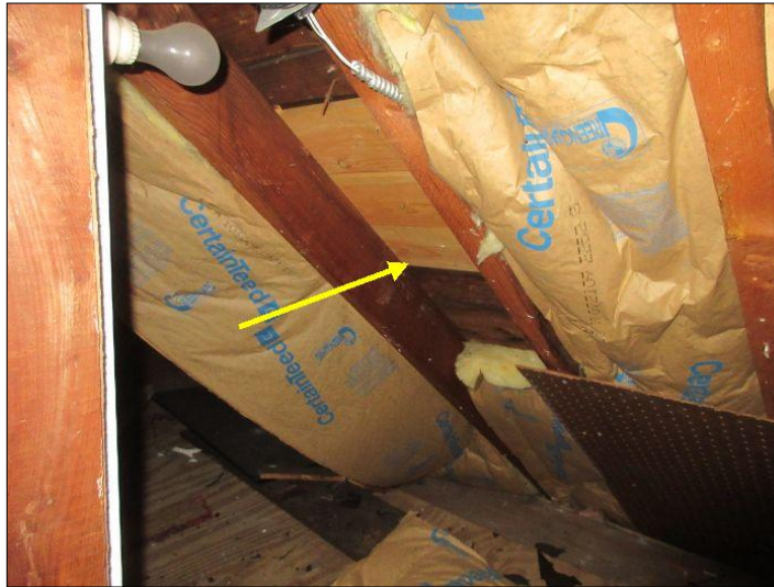
Loose insulation noted in attic area
