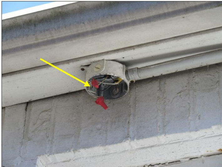
Light fixture missing. Exposed wires noted. (Left side)
