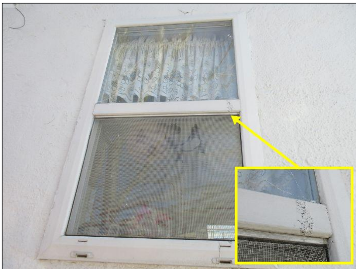
Deteriorated exterior finish noted (Right side)
