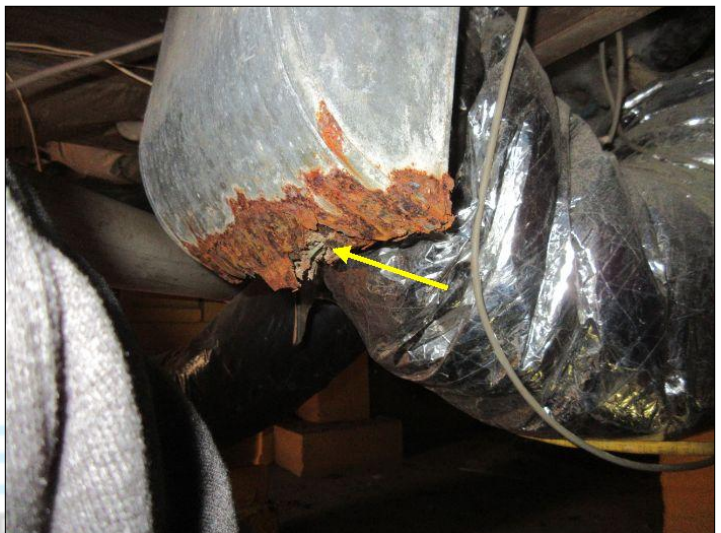
Rotted duct noted (Crawlspace)
