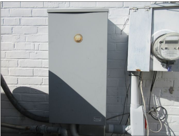
Backup generator disconnect
