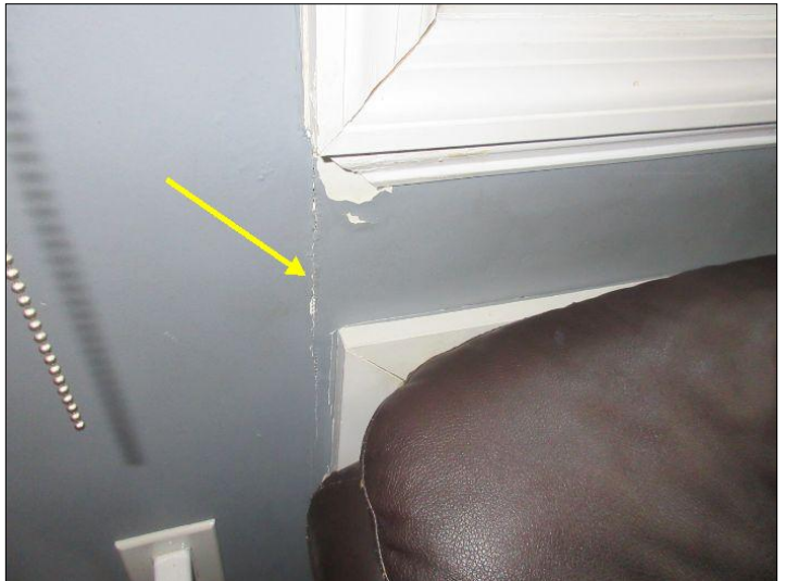
Damaged drywall noted (Bedroom #6)
