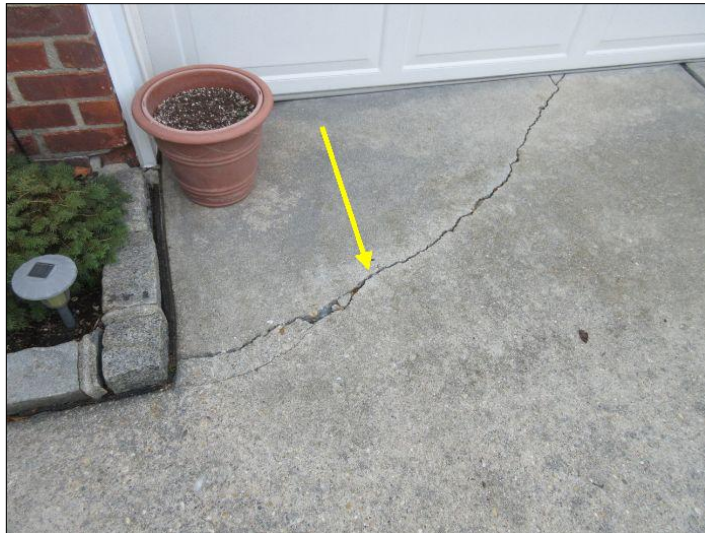
Common cracks noted
