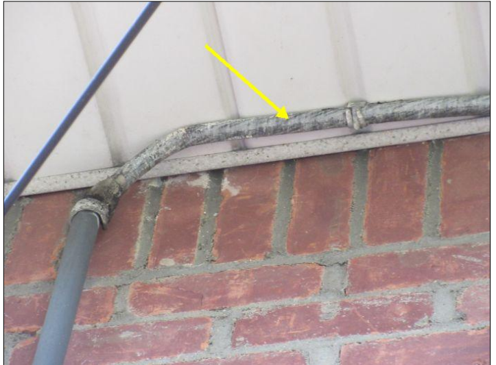
Sheathing on service entrance wires is in deteriorated condition. Recommend budgeting for upgrades to electrical service.
