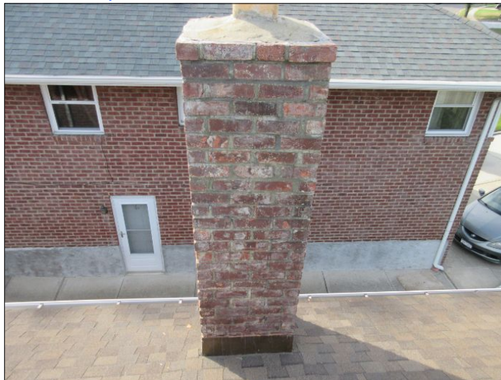
Appeared functional at time of inspection
