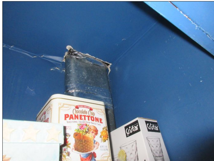
Exposed duct noted (Bedroom #3 closet)
