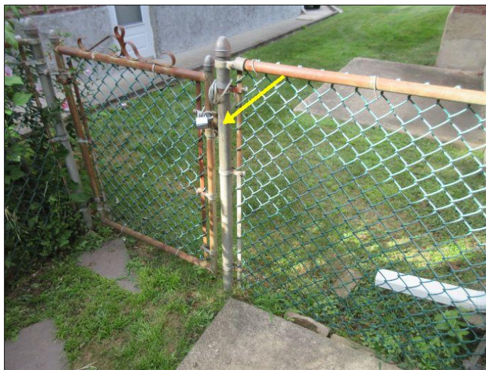
Gate requires adjustment
