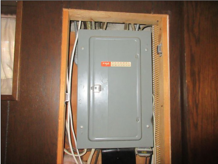
Recommend replacement during future renovations
