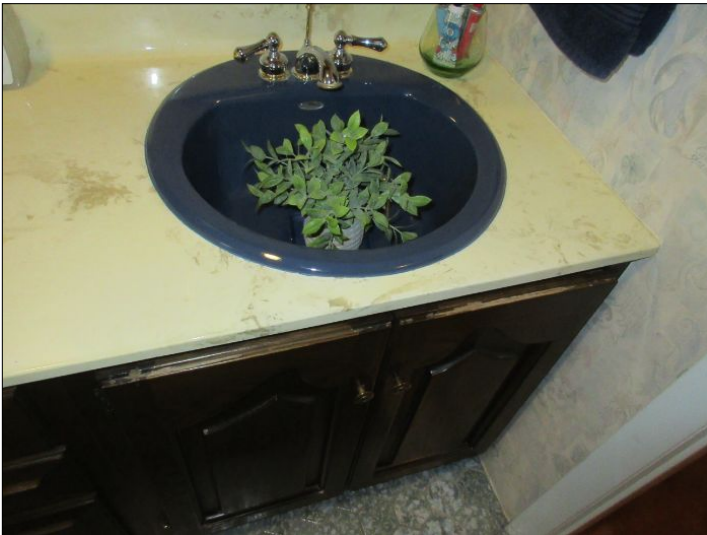
Owner stated right sink does not operate - Not tested
