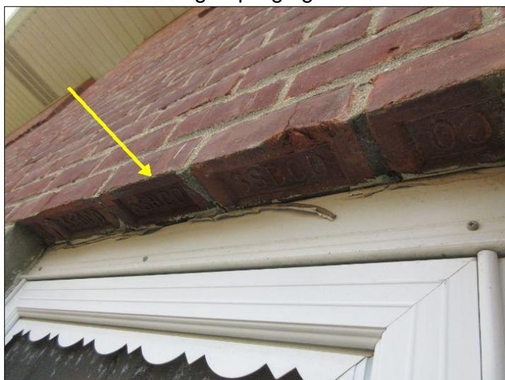
Missing lintel noted at doorway opening (Garage)
