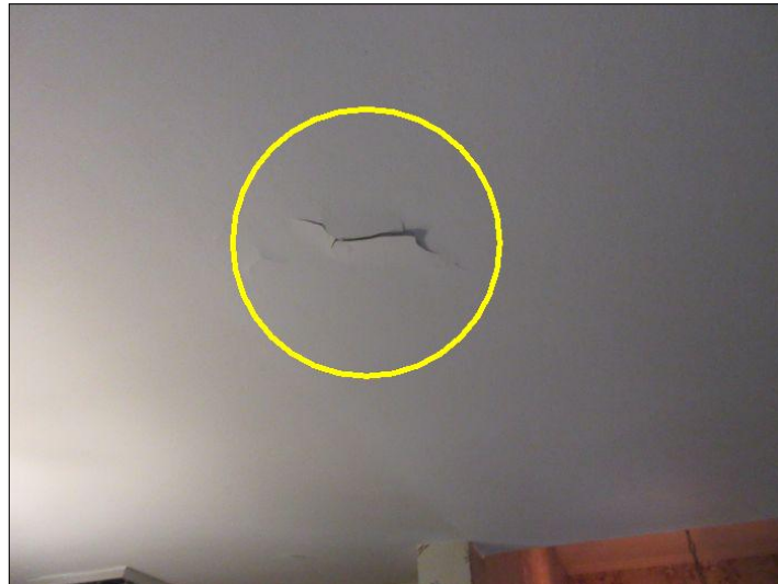
Peeling wallpaper noted (Kitchen)
