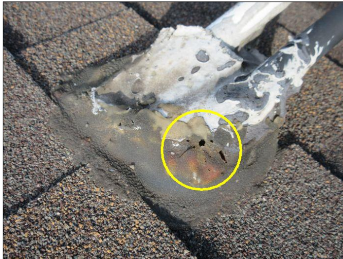
Recommend sealing as needed (Condensate drain)
