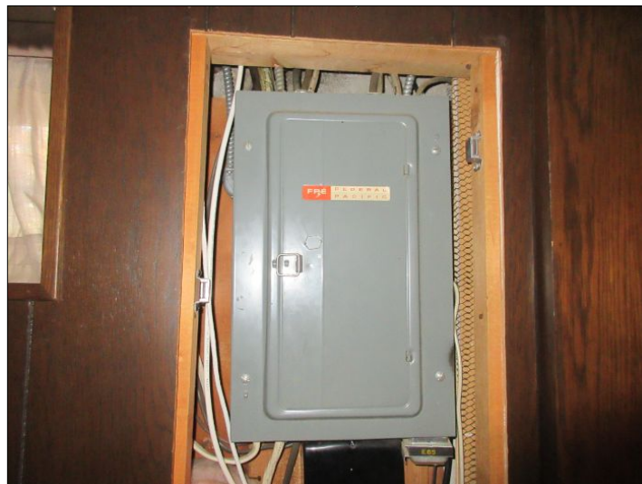
Recommend replacement during future renovations
