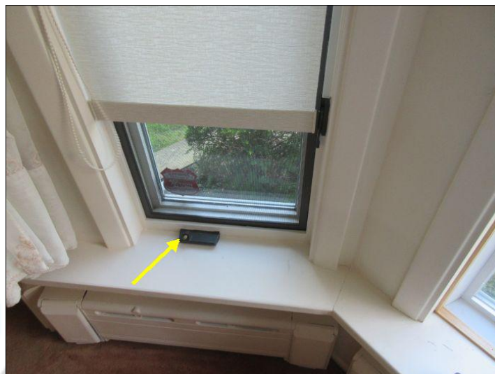
Missing handle noted
