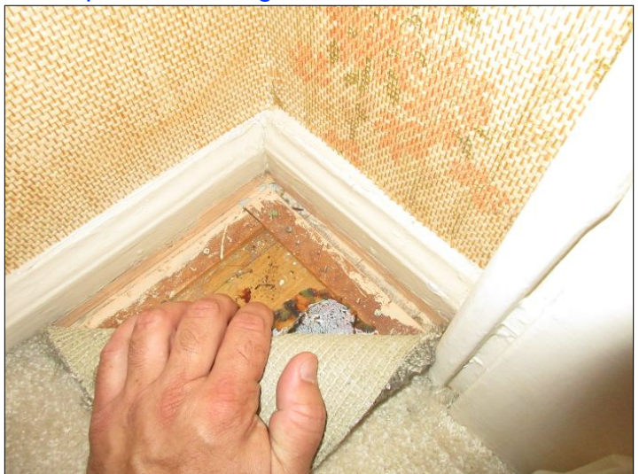
There are areas of hardwood flooring under carpet. Unable to fully evaluate.
