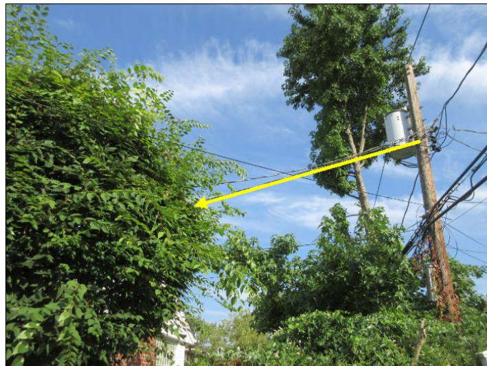
Wires are touching trees, recommend review by the local Utility Company for trimming as necessary.
