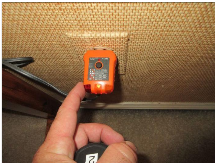
Open ground noted
