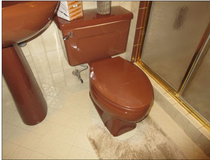
Operated when tested. No deficiencies noted.
