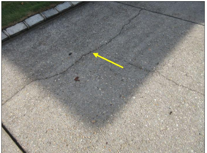
Common cracking noted
