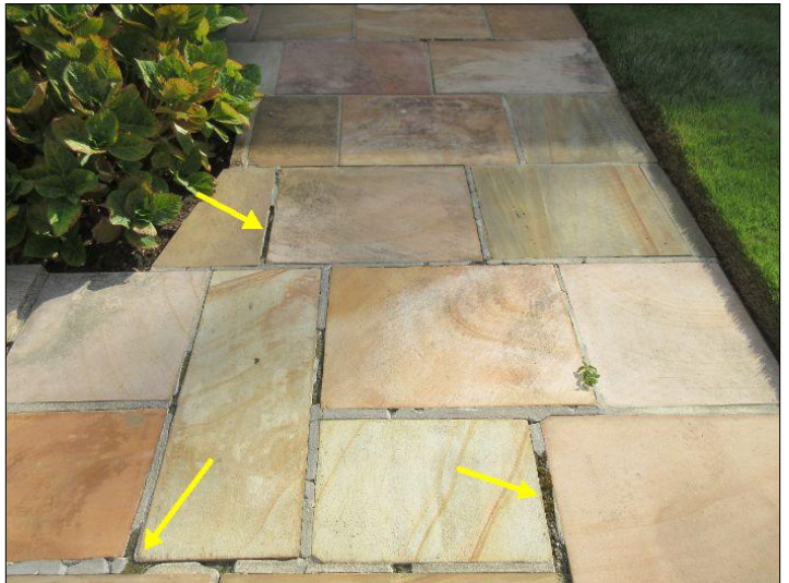
Some mortar joints require repair
