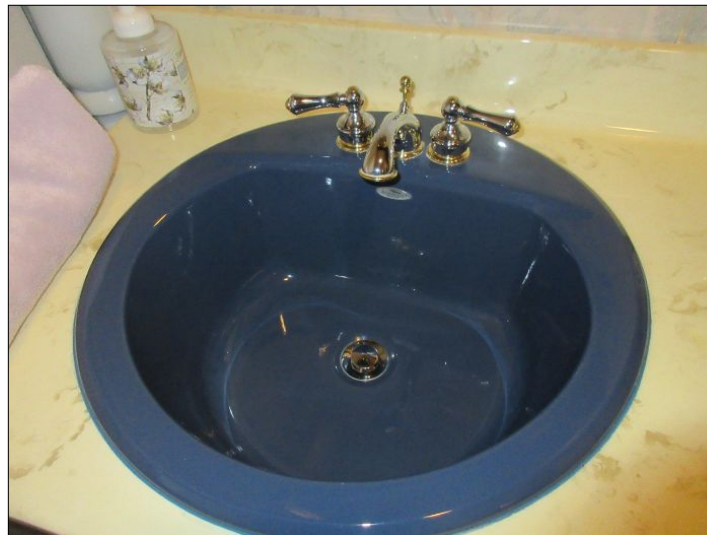
No deficiencies observed (Left sink)
