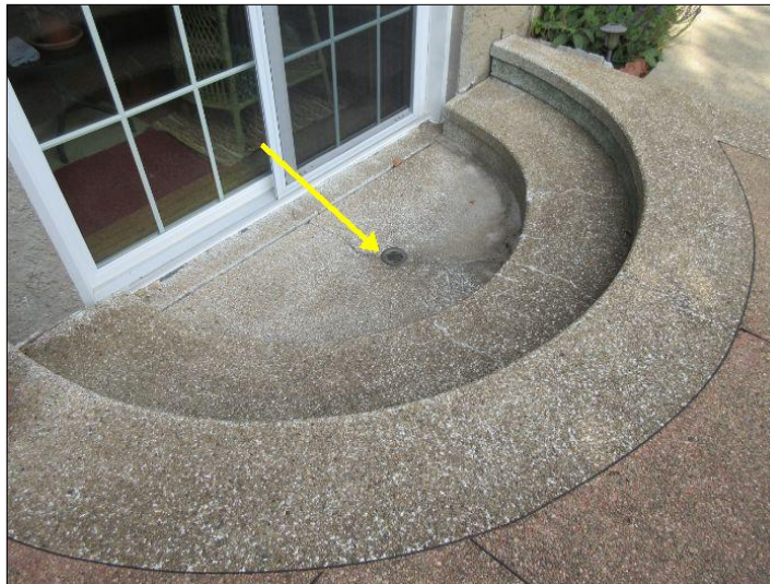
Maintain area free of debris to prevent clogging / flooding
