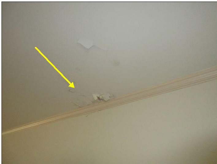
Blistering noted - Area did not appear wet when tested with moisture meter - Recommend monitoring (Living Room)
