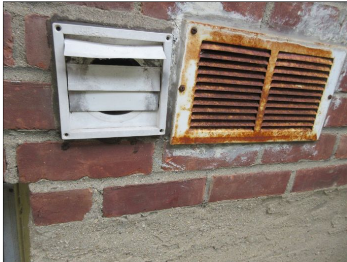
Properly vented to exterior
