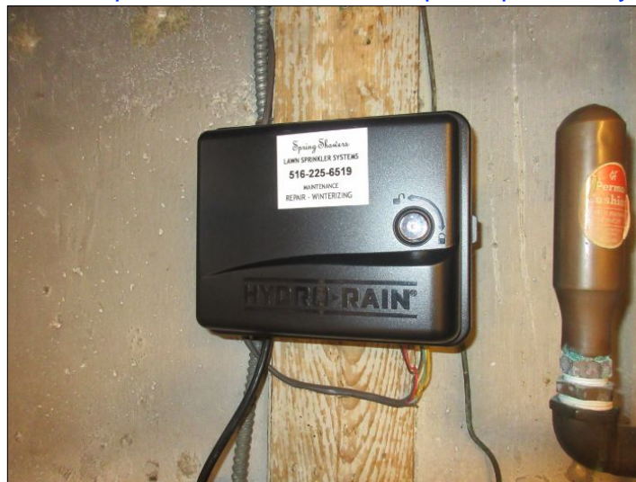
Sprinkler system timer
