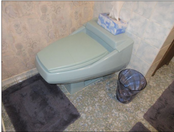
Operated when tested. No deficiencies noted.
