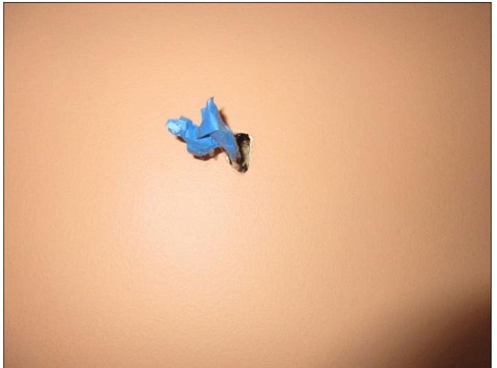
Exposed wiring noted from removed wall sconce. Recommend securing by licensed electrician (Living Room)
