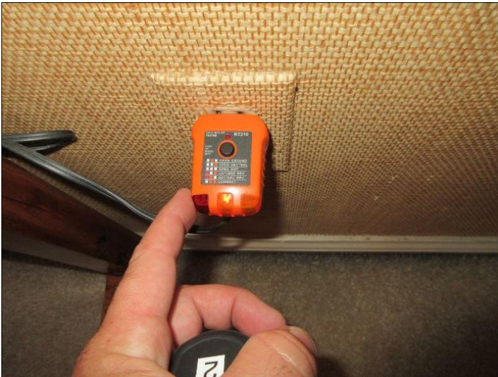
Open ground noted
